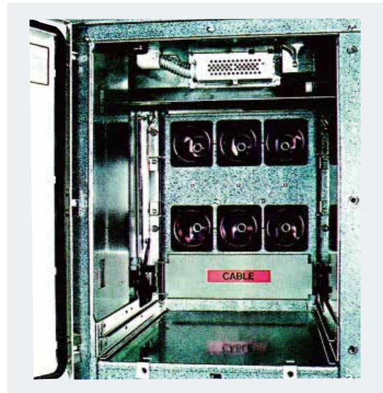
在断路器隔室内，打开金属活门检查静触头 Open the metal valve to check the static contacts inside the circuit breaker room
